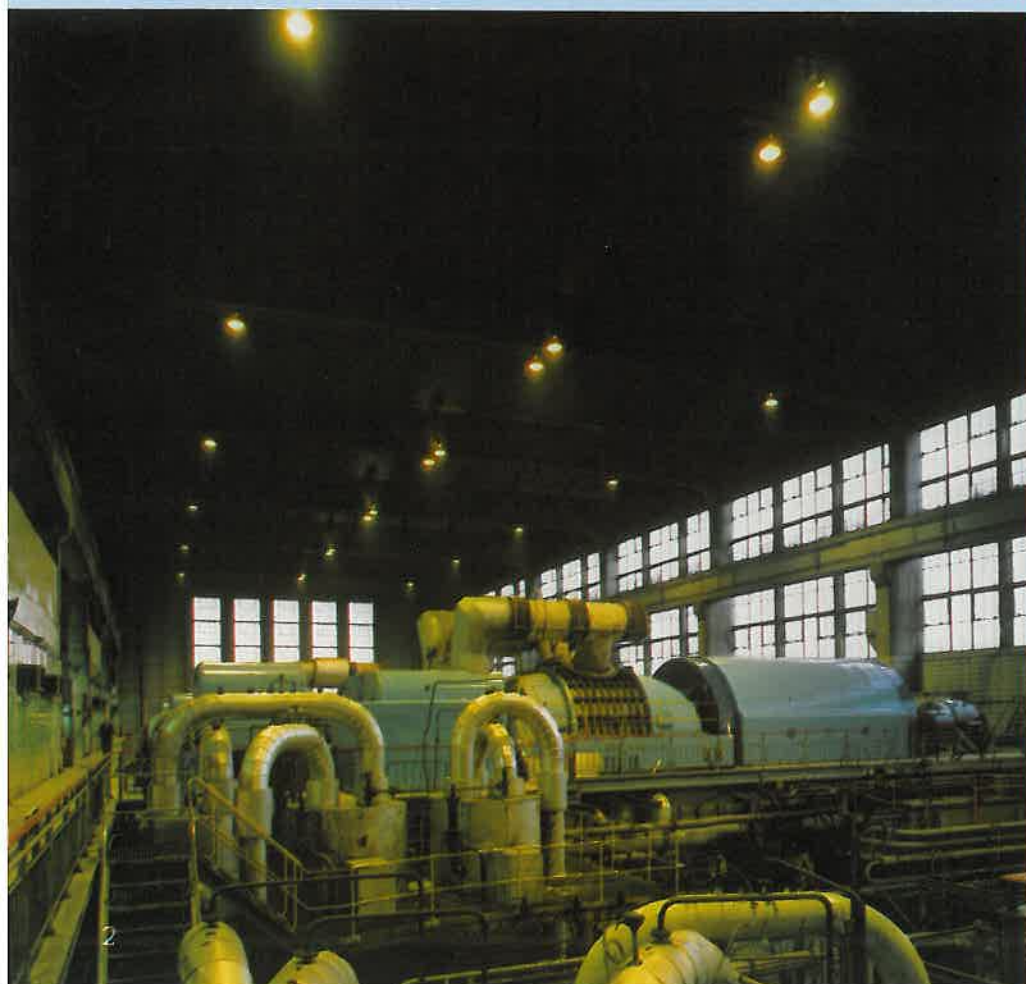
The turbine room of Skelton Grange CEGB generating station in Yorkshire. The forty 400W SON lamps are in use day and night as can be seen from the picture. Only half a dozen have failed in over 8,000 hours' use.
